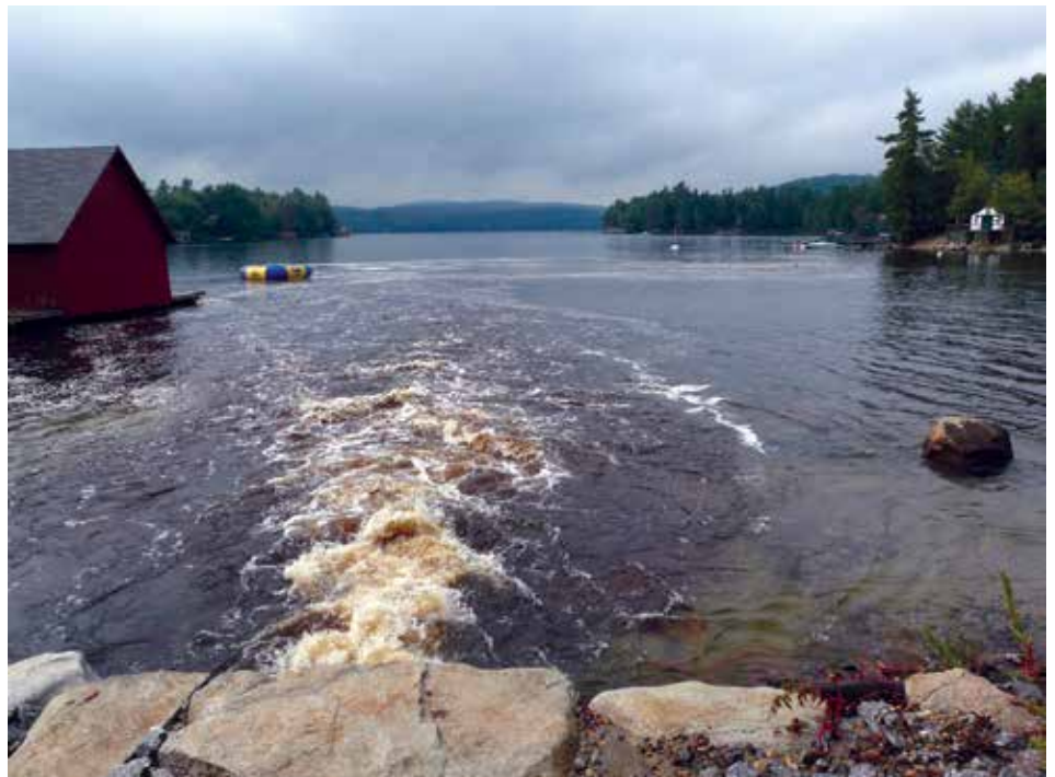
Figure 5. Stormwater flowing into Lake Sunapee, New Hampshire, through a road culvert. Photo: Midge Eliassen.
